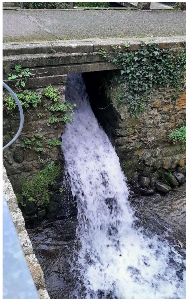
Figure 3 Rain Drain (SWO)
