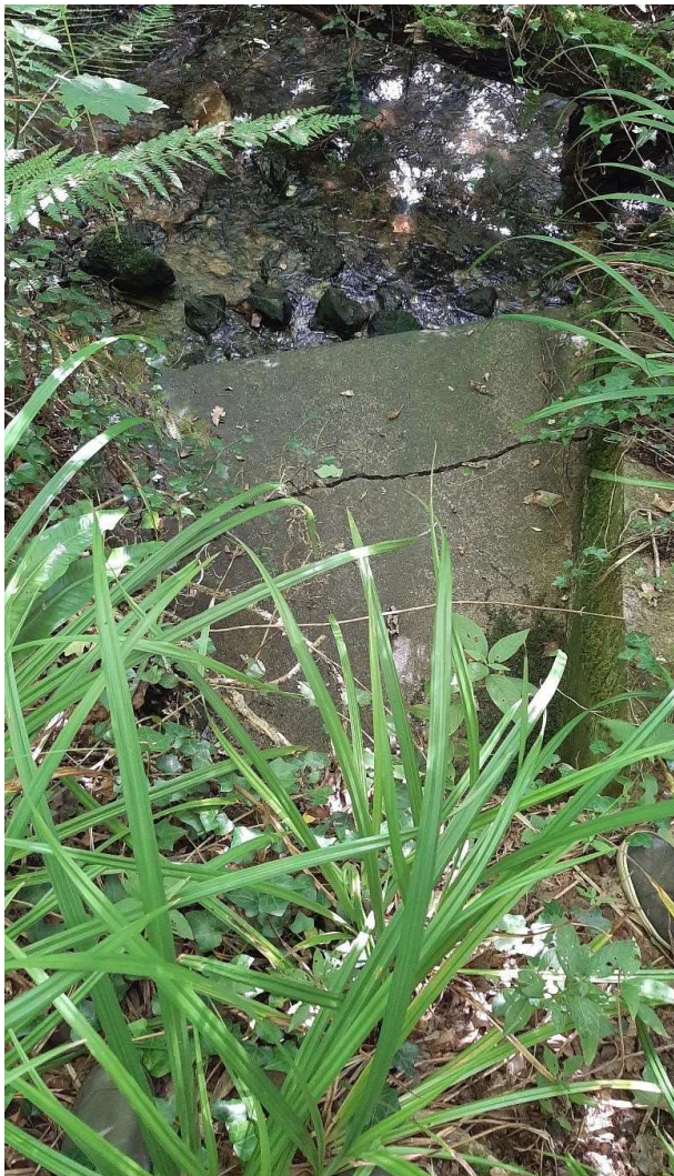
Figure 2 Sewage works CSO
